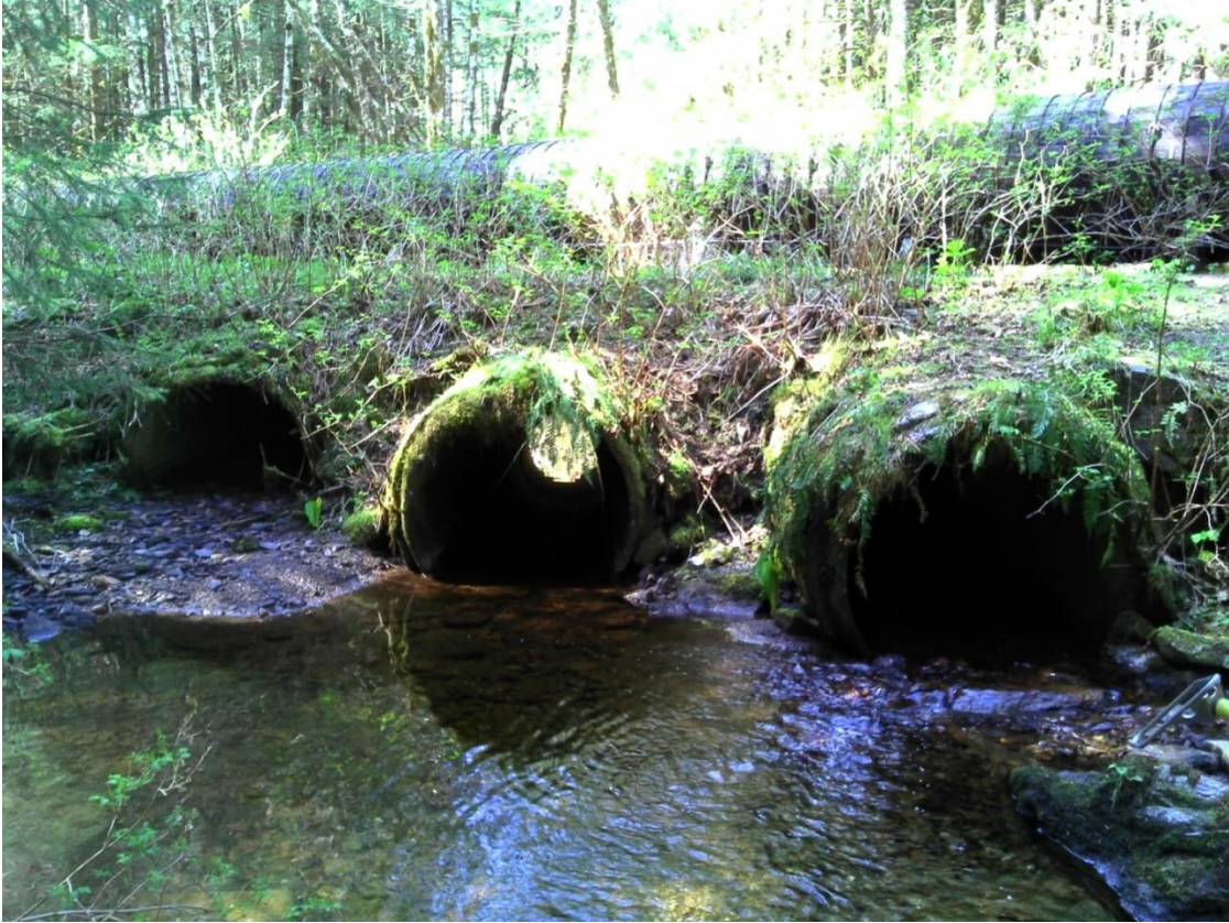
Figure 1.—Battery of three culverts under the Connell Lake penstock.
